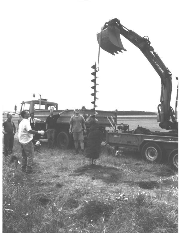
Figure A.1: Borehole drilling with a spiral drill ( Stihl, 2001 ), tiltmeter position T4_{OE} , see Fig.3.3 . The borehole is at the right side of the photo in front of the excavator. The spiral drill can also be operated by a drilling car.
